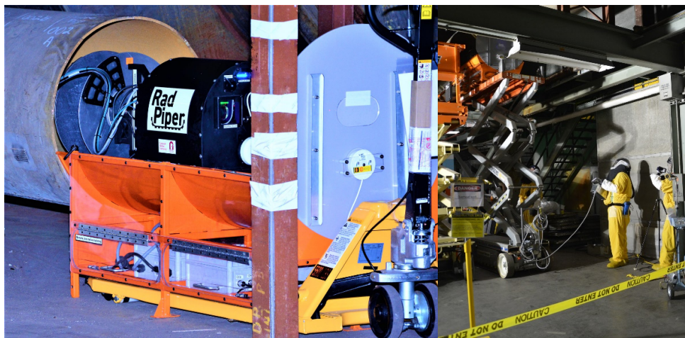
Fig. 12. RadPiper deploying into a (left) at-grade process pipe and (right) an elevated pipe.
