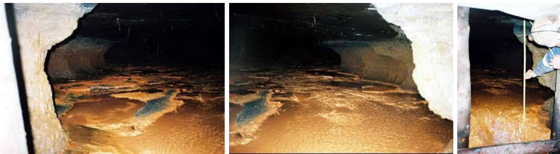
Figure 3.6: Breach between Quecreek and Saxman mines through which flooding occurred.
