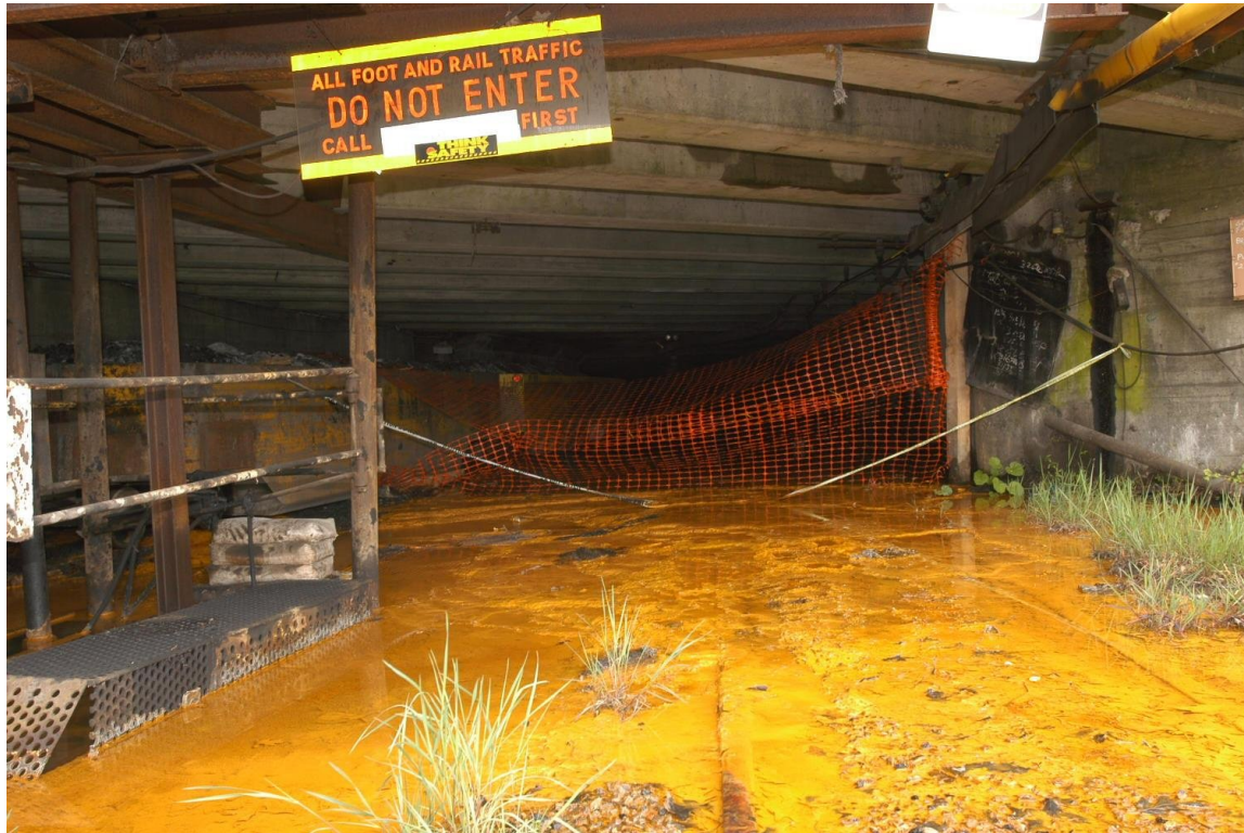
Figure 6.17: Wet, muddy conditions found at the downstream Mathies portal.
