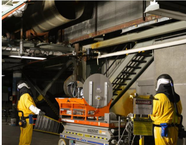
Fig. 2. (Top) Phase 1 RadPiper PCAMS robots undergoing testing at DOE Portsmouth. (Bottom) A RadPiper robot deploying in a Portsmouth process pipe.
