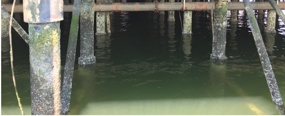
Figure 1.1: Pilings underneath a pier. The spacing between each pair of piles can differ and piles might be slanted.
